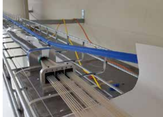
An 8-metre long prototype fibre cable has been constructed to test fabrication techniques and verify performance as a function of different environmental factors. Each individual optical fibre is slid inside a Teflon tube for protection and each of those tubes is held by a shear clamp at the ends of the cable (pictured here).
